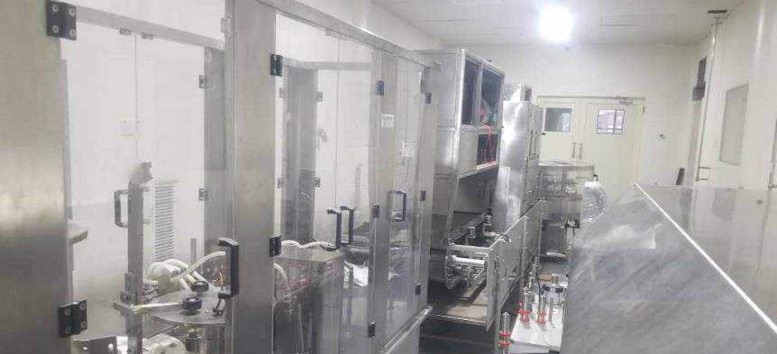
Packaging machines installed including washing, sterilization, fill and packaging, labeling and inspection machines
