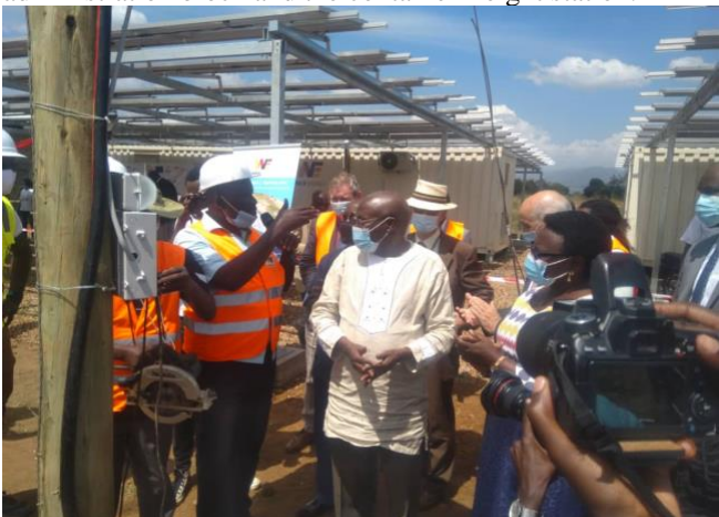
Solar PV Generation and storage systems in Lamwo under mini grids construction
