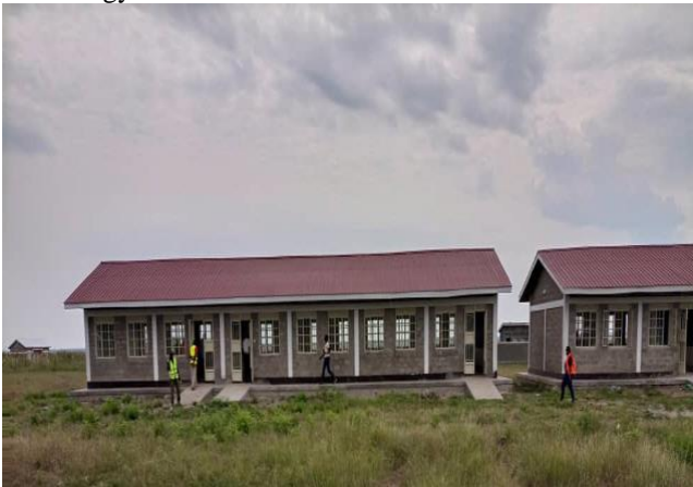
Classroom blocks constructed at Bunambutya settlement for disaster victims from Elgon sub-region
